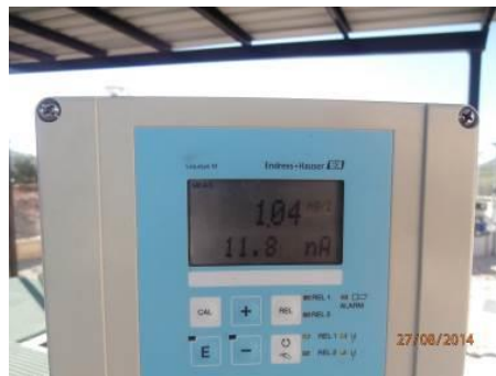
On-line sensors of Chlorine and Redox with alarms
